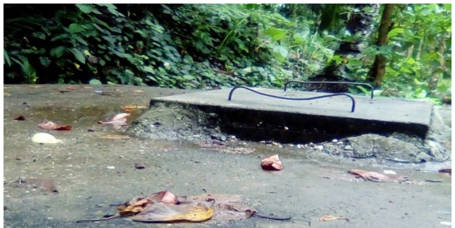
A ferro-cement water storage used by the local communities. Project officers along with zone representatives, conduct physical checks on community water sources and storage. All information feeds into the risk and hazard identification process and feedback from zone representatives to households. Image credit: Water for Women, Solomon Islands
